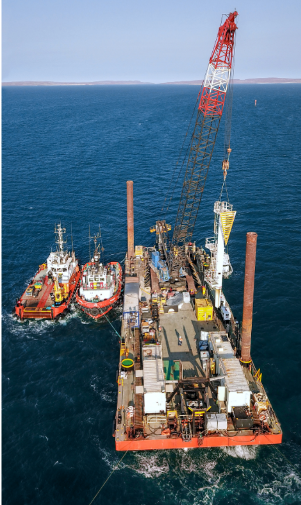
Recovering redundant Navigation Aid to the deck of TAMS9 Construction barge, with TAMS ANNEMARIE (Multicat) and PEGASUS (Tug) alongside.
