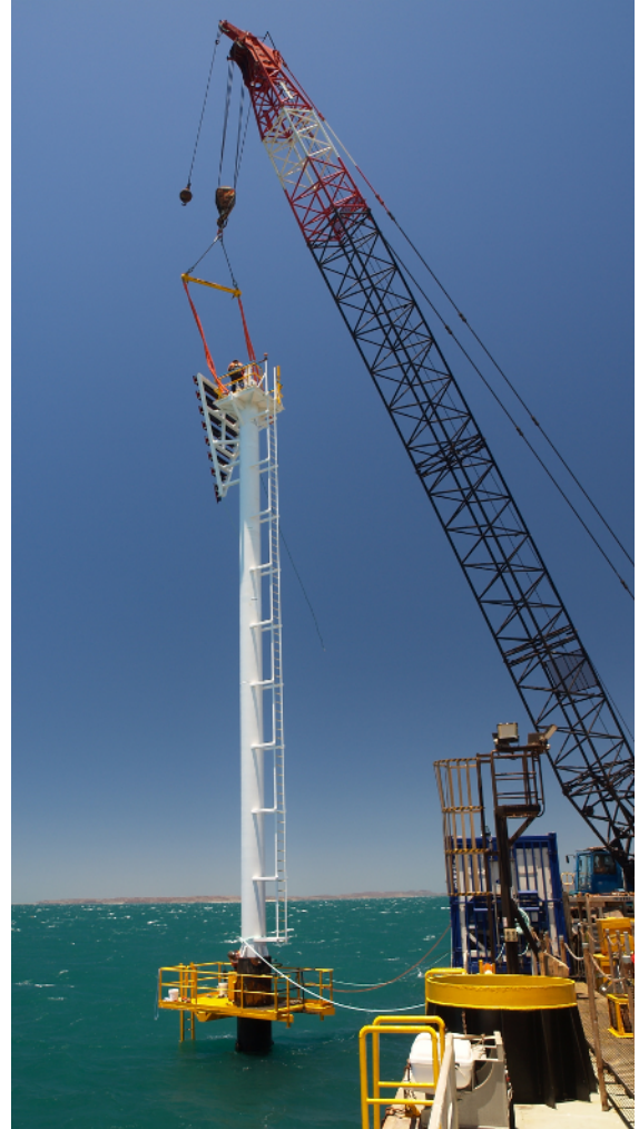
Installation of replacement topside structure with temporary access platform in place to support pile protection system application
