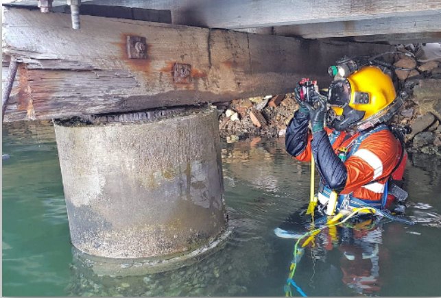
Diver takes still photos of existing timber pile protection interface to crossheads
