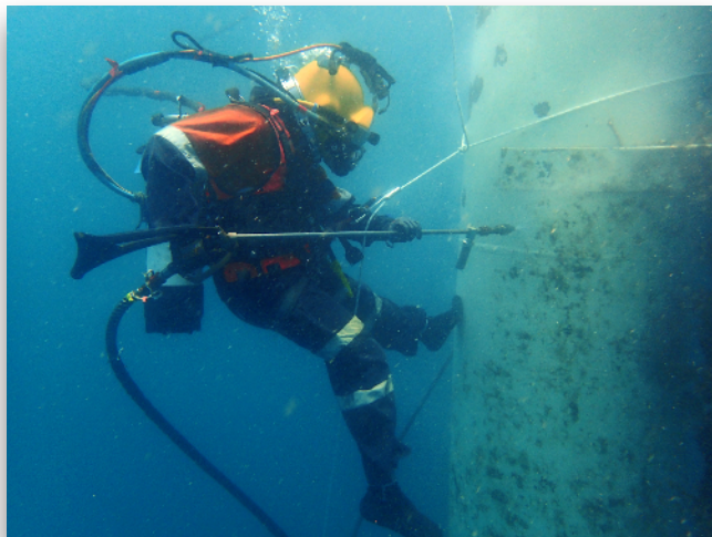
Diver prepares pile surface with high pressure water blaster to facilitate a detailed coating inspection
