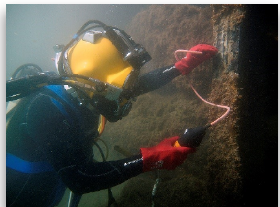
Diver obtains steel thickness readings of steel sheet pile wall using ultrasonic thickness meter.
