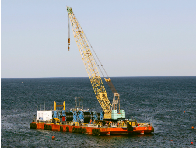
TAMS crane barge in mooring spread ready to lay dual high pressure hydraulic pipelines from 3.5 km offshore.
