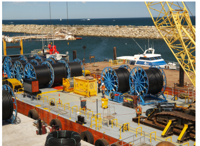
Mobilisation of barges at TAMS Fremantle shore base, utilising wharf and onshore facilities, plant and labour.
