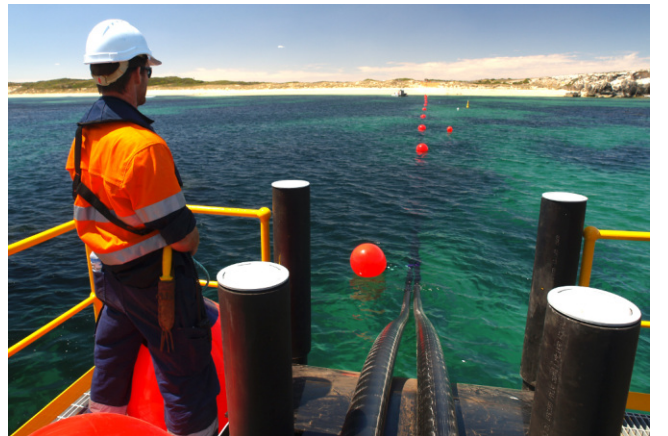
Shore-pull to onshore plant through pre-installed conduit, using a fully integrated service offering.
